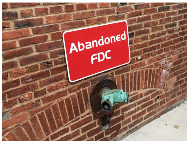
Fig. 1. A nonworking standpipe (left in place for historical reasons) is signed so that fire companies will not attempt to use it in an emergency (Baltimore, MD).
